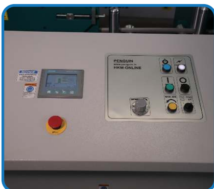
Control panel with PLC
